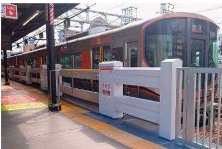
Improved movable platform screen doors Jointly developed by West Japan Railway Company, West Japan Railway Technic Co., Ltd., and Naitesco Corporation
