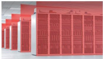
Server rack protection
