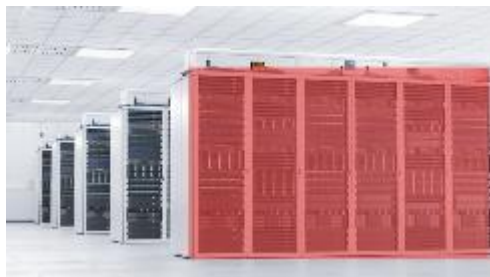
Example of intrusion detection in a data center
