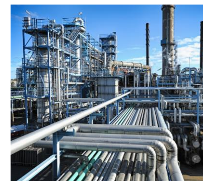
Oil, gas, and other infrastructure facilities
